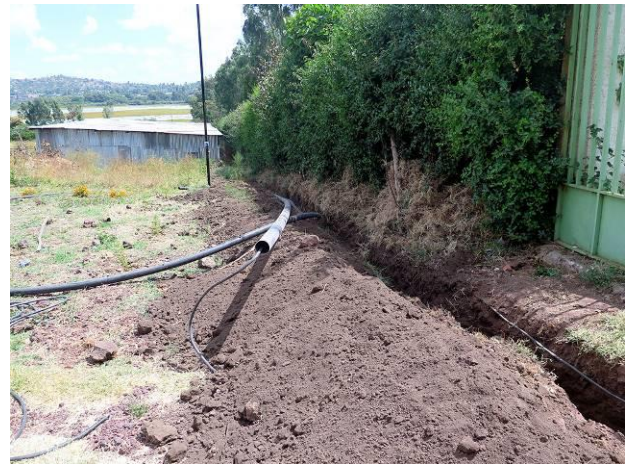
pipeline from well to tank
