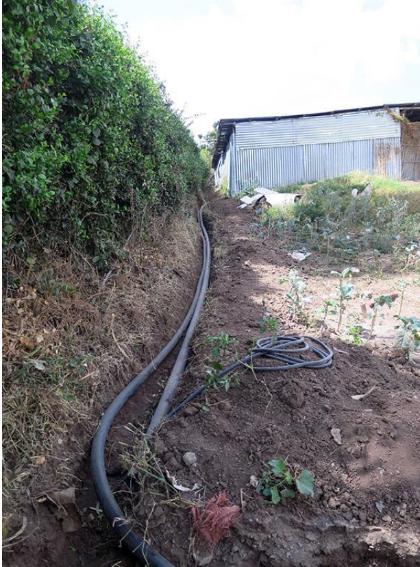
pipeline from well to tank
